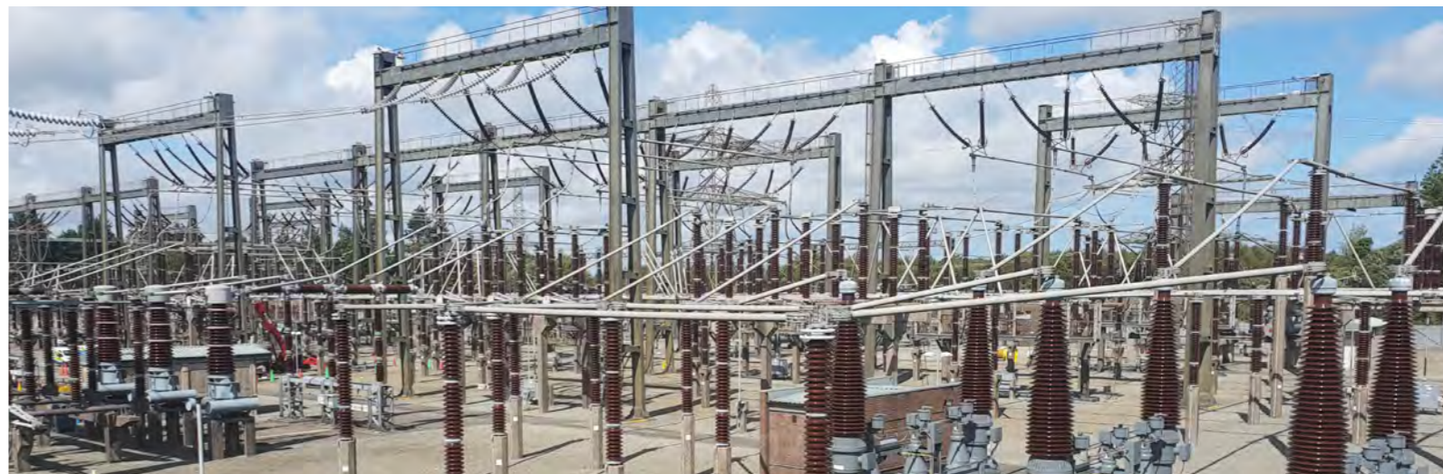
Existing Pentir Substation
